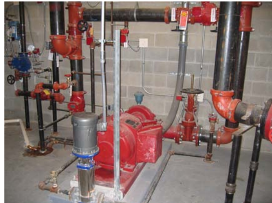
Fig 13 – Fire Pump Room
