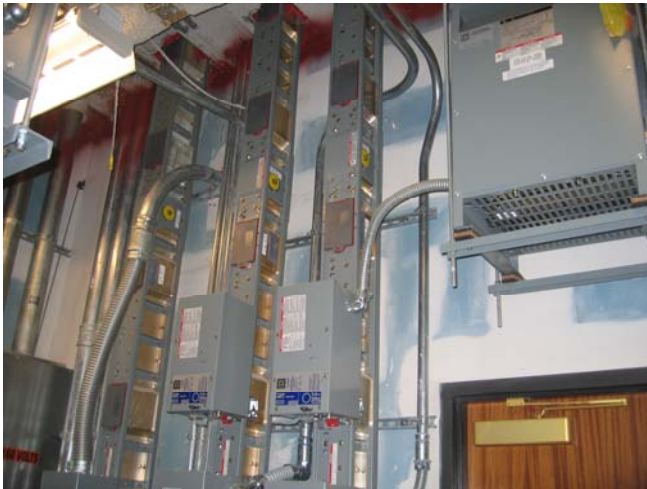
Fig 5 – Typical Floor Electrical Rm showing bust ducts and a transformer
