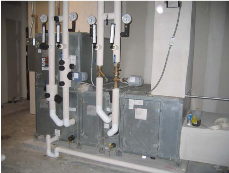
Fig 7 – Mechanical Room showing Air Handling Unit
