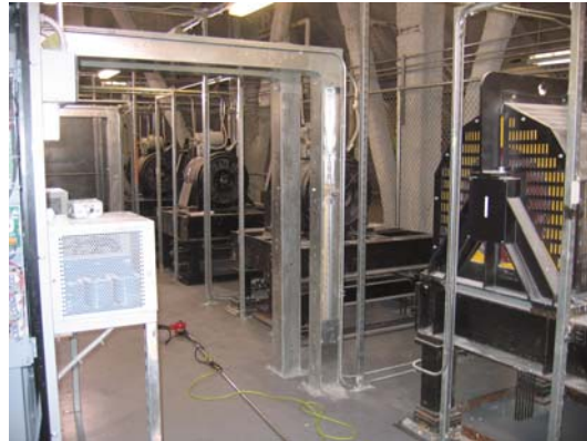
Fig 14 – Elevator Machine Room
